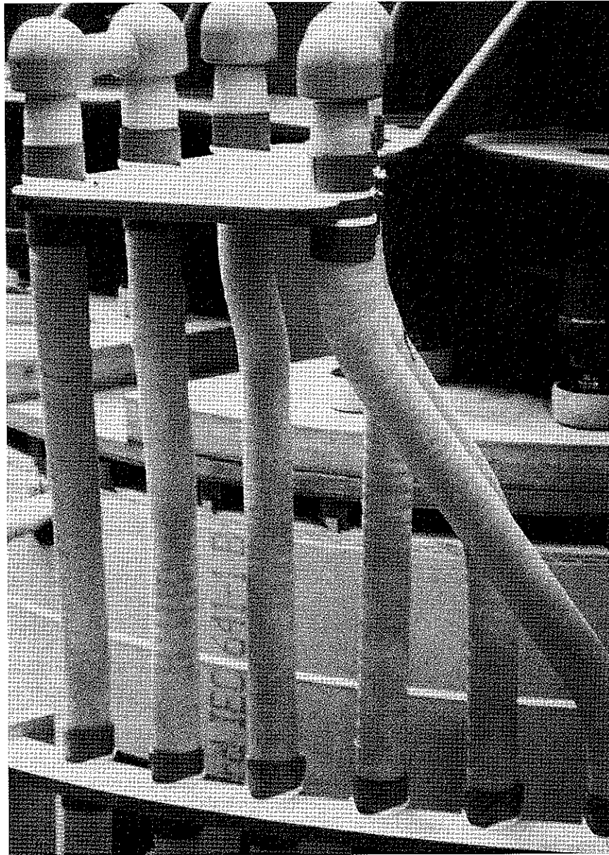
Figure 4.66 Arrangement of links under oil used to provide off-circuit taps on the HV winding of a 650 MVA, 20.9/345 kV, generator transformer supplied to the USA (Peebles Transformers)
